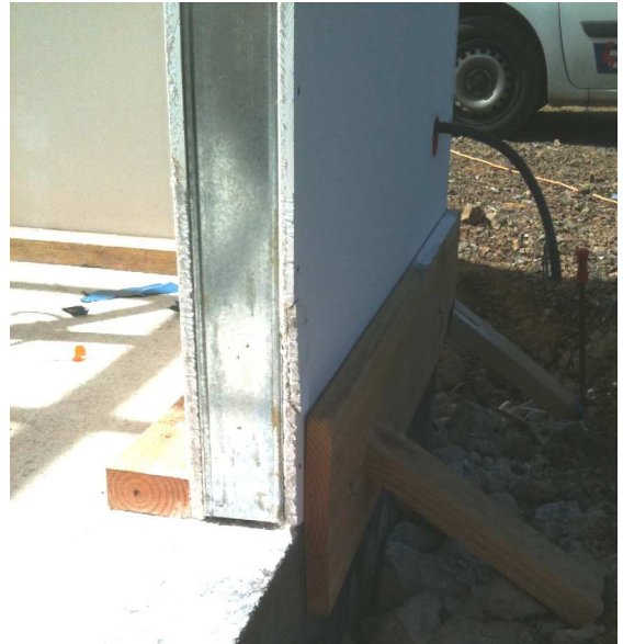
Whale boards positioned to assist panel placement with external concrete fill supports
