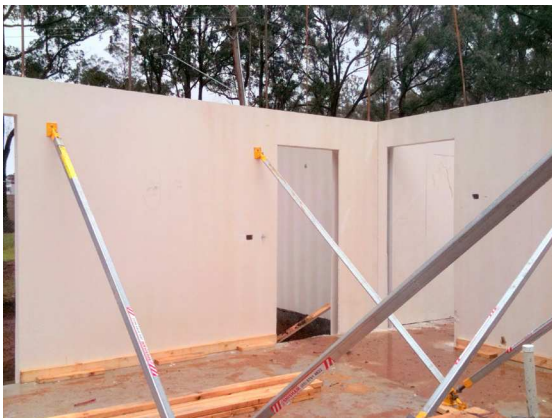
Props in position, note 'whale' boards also installed to assist in positioning panel
