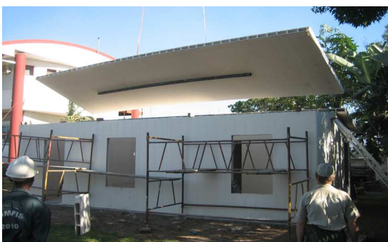
Sequence of photographs showing lifting of roof panel into position with under panel spreader bar
