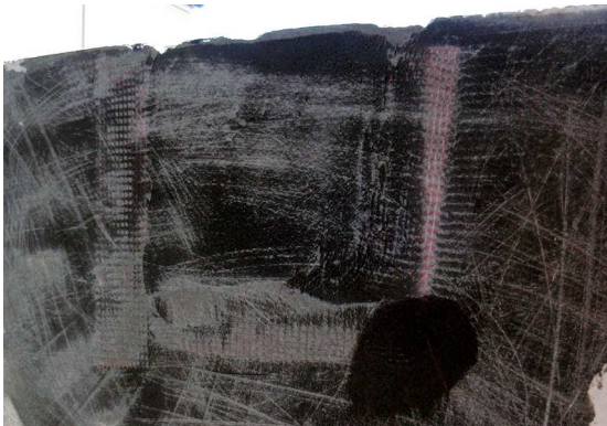
Repaired section of panel showing fibre glass tape, patching plaster and primer
